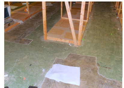
Fig. 2—Floor tile containing asbestos
