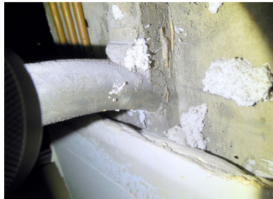
Fig. 1—Asbestos was found in the pipe wrap
