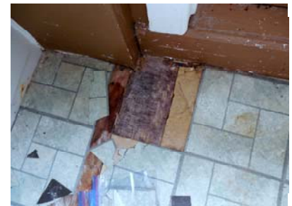
Fig. 2—Asbestos identified in vinyl floor tiles
