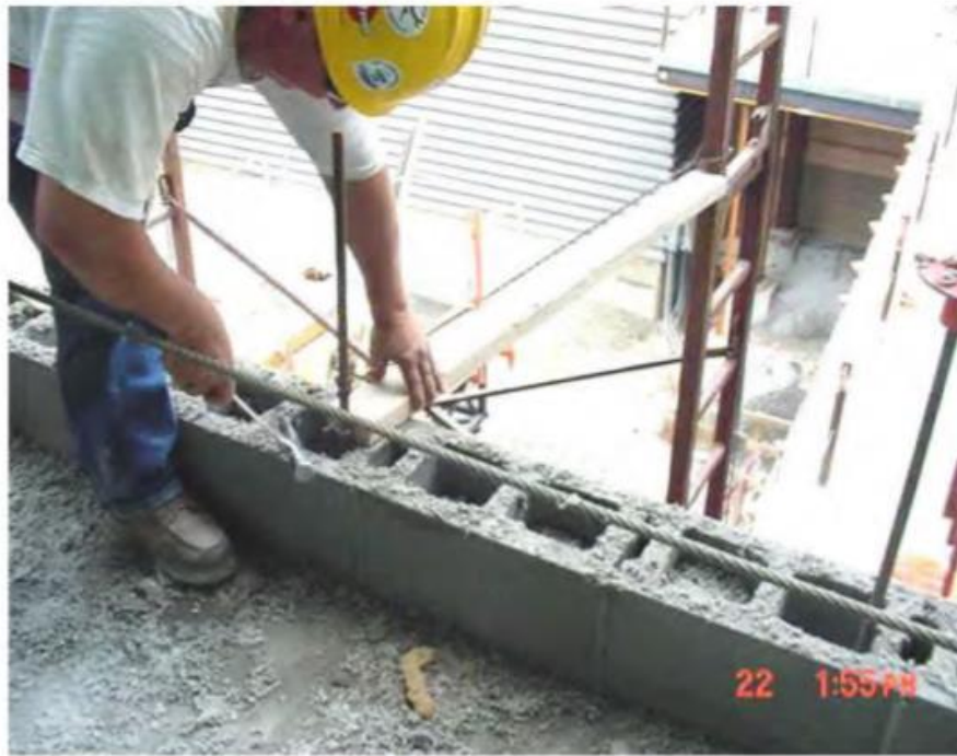
Protection often removed to work
