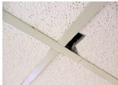
Fig. 1—Analytical testing confirmed the ceiling tiles contained asbestos
